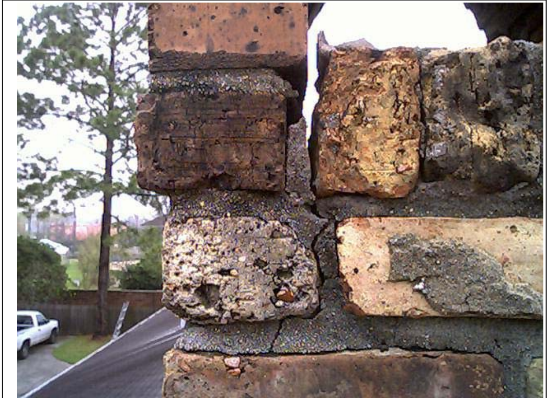
Mortar joints are deteriorated, Improper clearance to combustibles.
